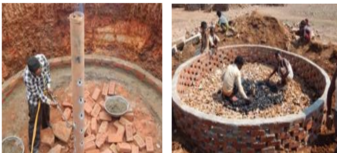
Figure 10 Locally made and cost effective solution, using old dry wells as recharge wells.
